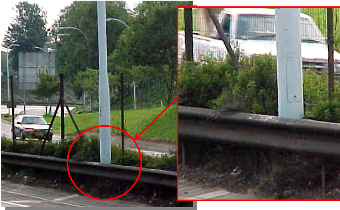
This lighting pole is located within the clear zone. Although it seems to be protected by guard rail there is no deflection distance available and could result in pocketing when impacted.
