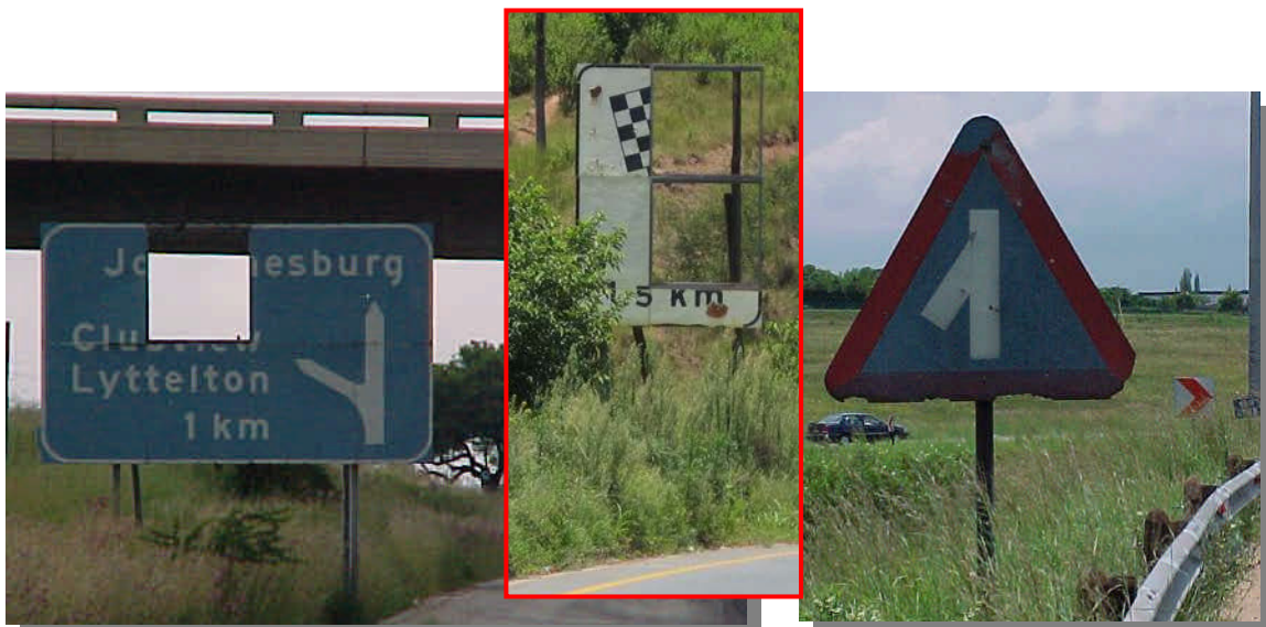
Worn and damaged road signs that provide little warning or guidance to motorists.
