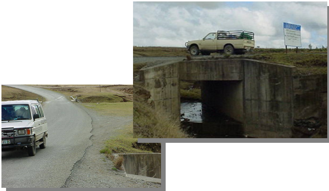
Two views of the same culvert to show the high risk situation when appropriate traffic barriers are not installed
