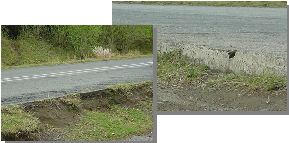
Examples of highly dangerous edge drops between traffic lanes and shoulders
