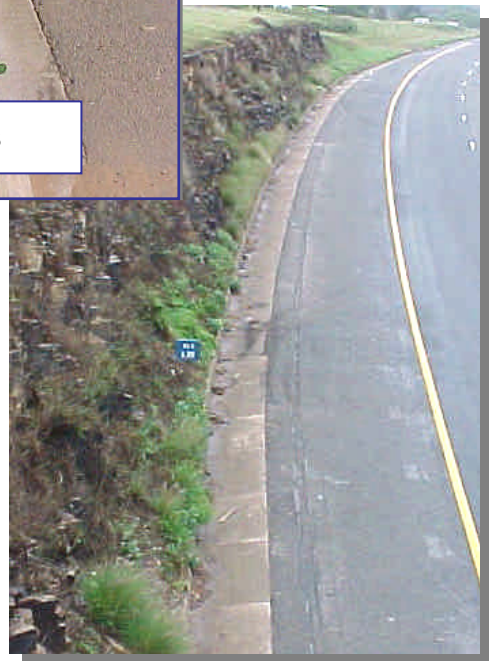
Back Slope Non - Traversable
